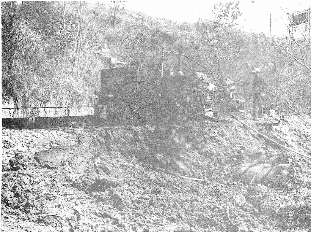
Figure 10. A Temporary Earth Fill had to be Constructed in order to Drill the Line of Holes Across the Top of the Culvert.
