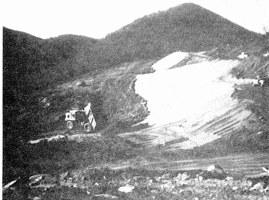
Figure 15. Embankment material being placed over sand and stone blanket. Lighter material is stone; the darker, sand.
