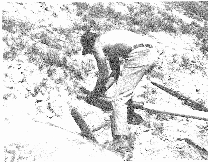
Figure 4. Air hammer on the end of the drill rod is being positioned to start a hole.
