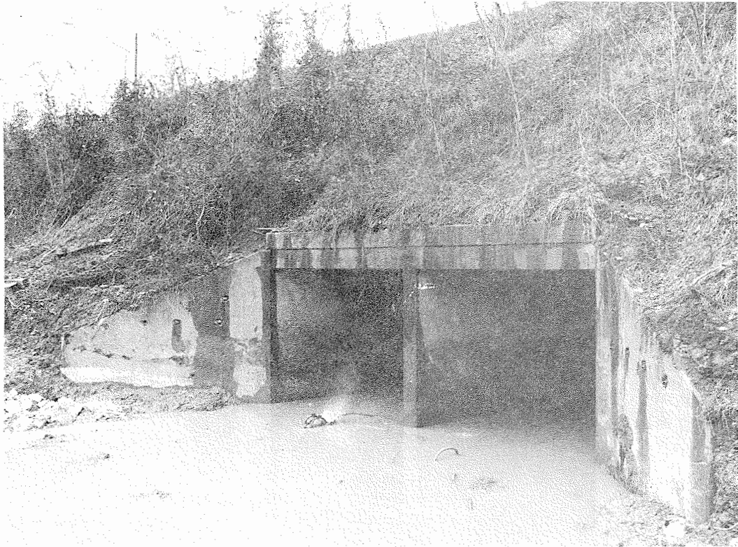
Figure 11. View of the Culvert After Completion of Drilling. Note Drains protruding from the wing walls and along the top of the Box.
