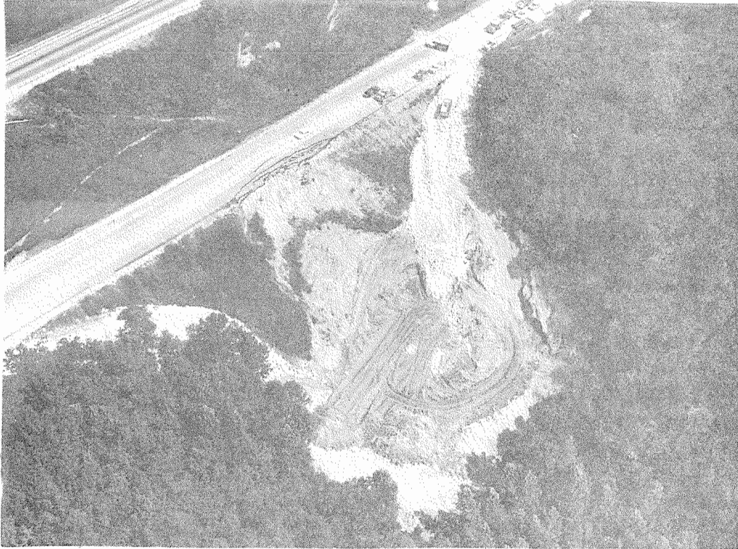
Figure 13. View of the 1464+00 slide along I-75 in Campbell County.
