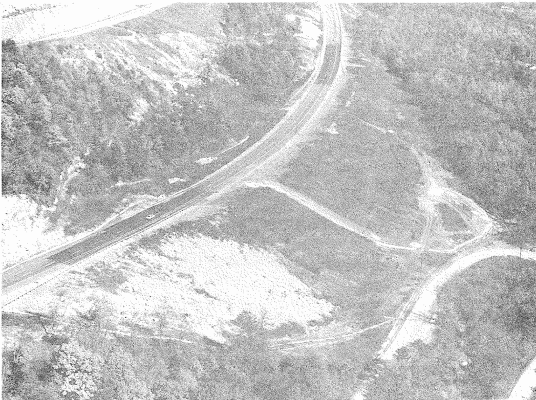
Figure 24. The 2003+00-2018+00 Fill Slide at Rockwood. Newly paved areas on each end of the embankment delineate the lateral limits of the slide.
