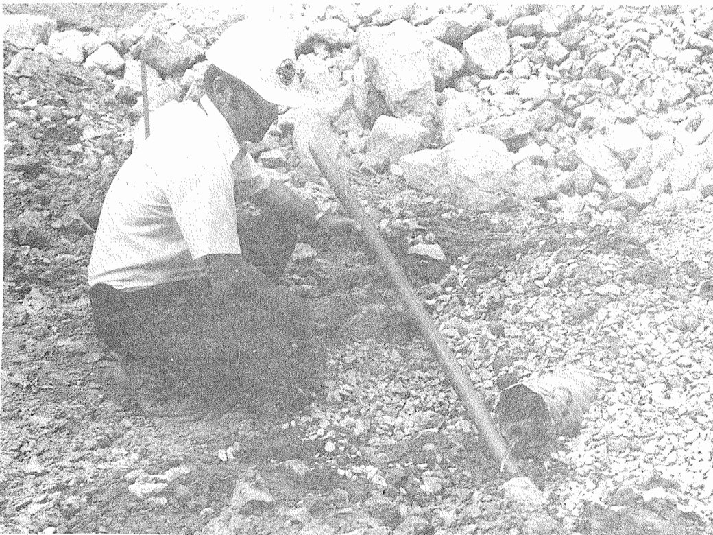
Figure 14. Water issuing from a Horizontal Drain installed in the 1464+00 slide.
