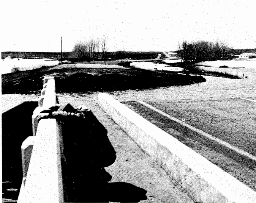
Figure 15. Photo showing erosion on the west end of Stone Bridge caused by water flowing from Dry Lake to Lake Poinsett (April 11, 1969).
