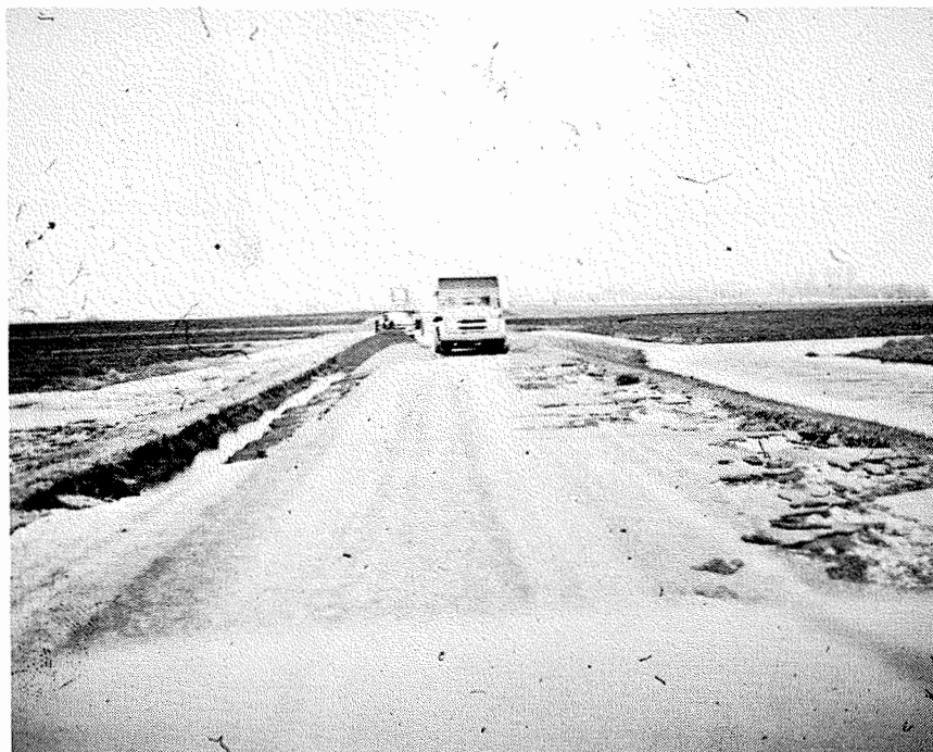
Figure 16. Photo showing repair of Castlewood Road after the flood of 1969 (3 miles north of Lake Poinsett).
